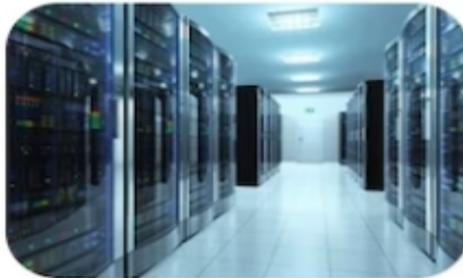
Giant servers used for cloud computing services
